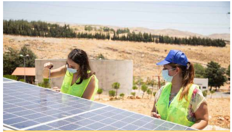
In Lebanon, women install solar panels as part of efforts to empower women in the renewable energy sector, improving their skills for economic empowerment during crises and the pandemic.
